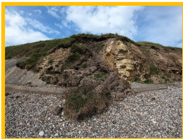
Minor outflanking of blockwork revetment and slippage at south end of seawall (/0102C01)
