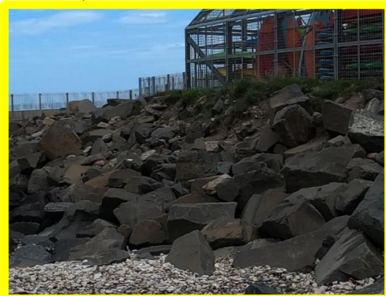
Low spot in revetment causing erosion to bank (/0104C02)
