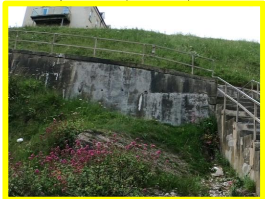
Cracking in retaining wall to access steps and ramp (/0103C07)
