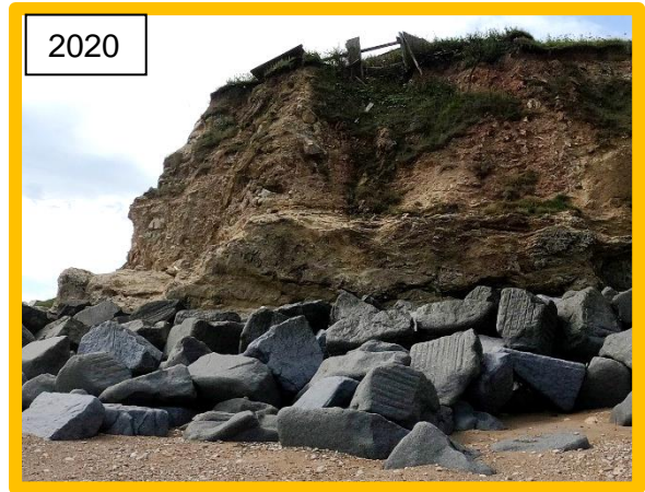
Erosion affecting fence line of properties to south Dawdon Dene Outfall - 2020 (/0103C02)
