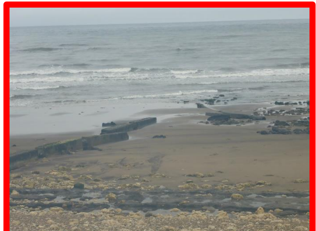
Failed section of concrete-encased outfall structure (/0201C01)
