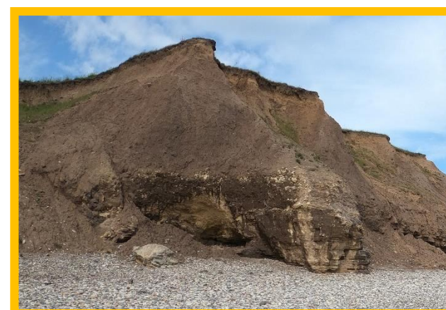
Localised slumping of upper till within the cliffs (/0804C01)
