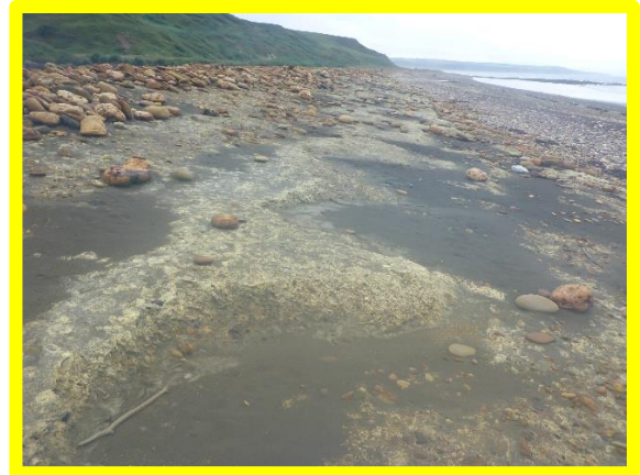
Minor erosion to colliery spoil to the south of the bay (/0201C02)
