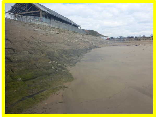
Open joints and vegetation growth on masonry revetment. High sediment levels (/0104C05)
