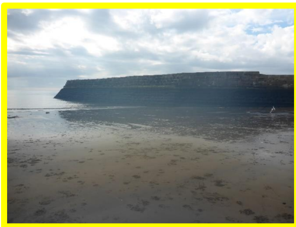
Inner Pier north face largely obscured by marine growth (/0104C06)
