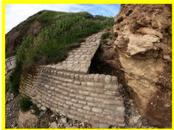
Outflanking of revetment (/0804C01)
