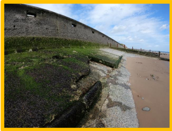
Failed section of concrete apron (/0102C01)
