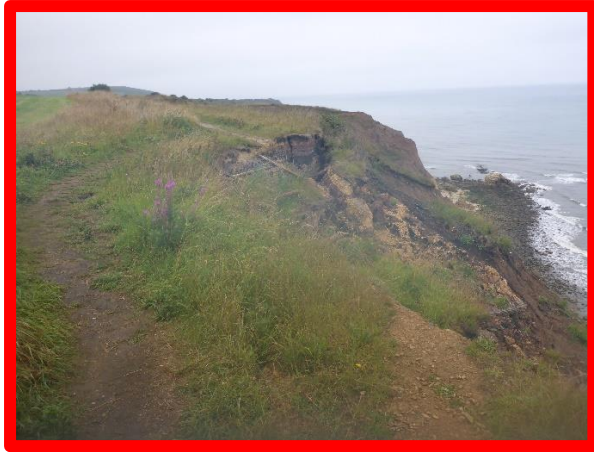
Cliff failure through coastal footpath (/0201C01)
