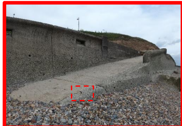
Hole in deck of ramp and exposed reinforcement (/0102C01)
