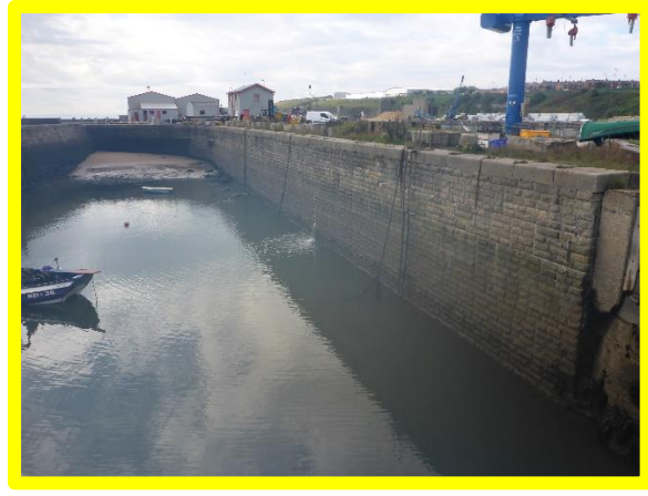
Inner face appeared in good to fair condition (/0104C10)
