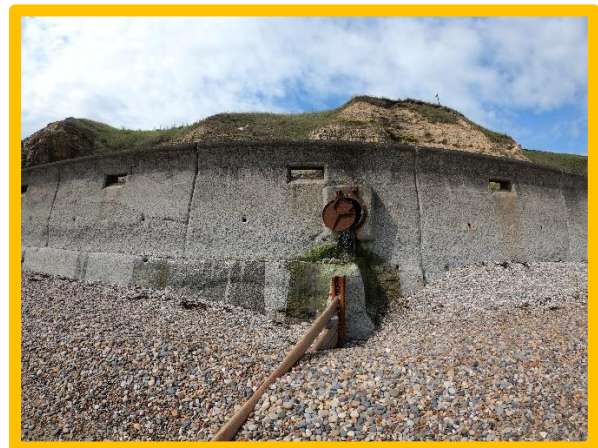
failed cast iron flap valve (/0102C01)
