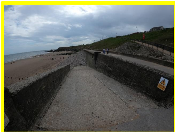
Cracks in deck of access ramp at southern end of promenade (/0102C01)
