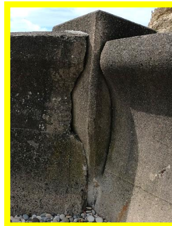
Sealant missing at joint between sea wall and access steps (/0102C01)
